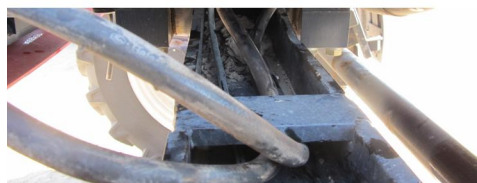
Figure 7a: Steering lines connected to run-tees, steering hoses reconnected, hoses routed towards the steering block
