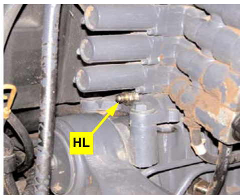
Figure 7a: Installed pressure fitting
