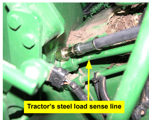
Figure 7a-ii: Tractor's steel load sense line at rear casting
