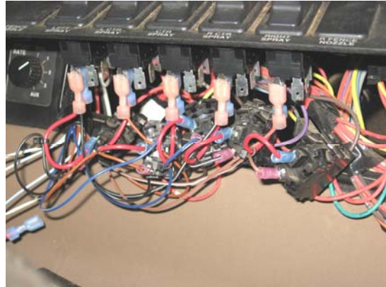
Fig. 6: Boom switches connected
