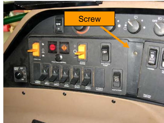
Fig. 1: Boom switch control panel
