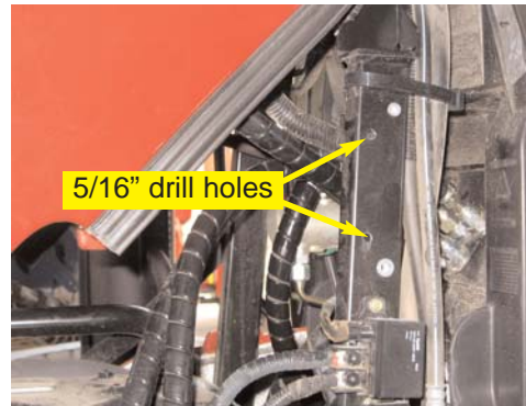
Figure 7a. Counter-balance valve location.
