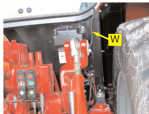
Figure 10c. Valve cable routed in cab.
