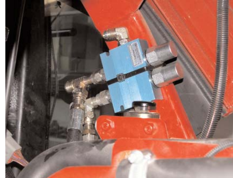
Figure 4b. Installed counter-balance valve block.
