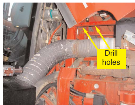
Figure 4a. Installed counter-balance valve block.
