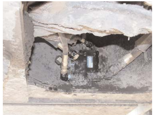
Figure 4c. Disconnected excess-flow line.
