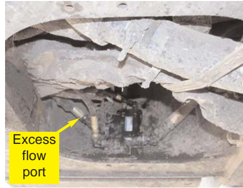
Figure 3a. Excess-flow location at priority valve.
