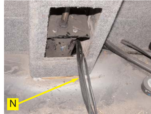
Figure 7b. Routed valve cable into the cab near the orbital.
