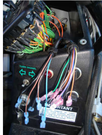
Fig. 3: Interface cable routing
