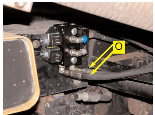
Figure 4b. Installed pressure and tank hoses at Automated Steering Block.
