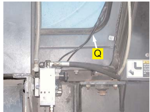
Figure 7b. Routed valve control cable.
