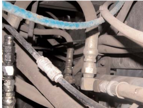
Figure 3e. Return manifold location.
