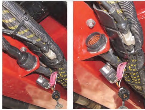
Figure 2a: Boom switch connection—before and after disconnection
