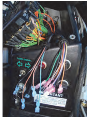
Figure 2c: Interface cable routing
