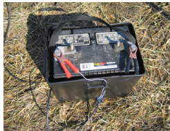
Power cable connected to battery
